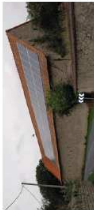
Roof equn - panneaux photovoltaïques
